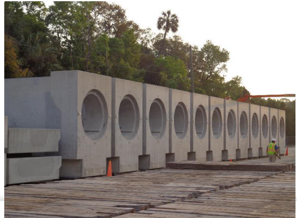
Horizontal Storage Modules Staged at Nuclear Spur after Unloading
