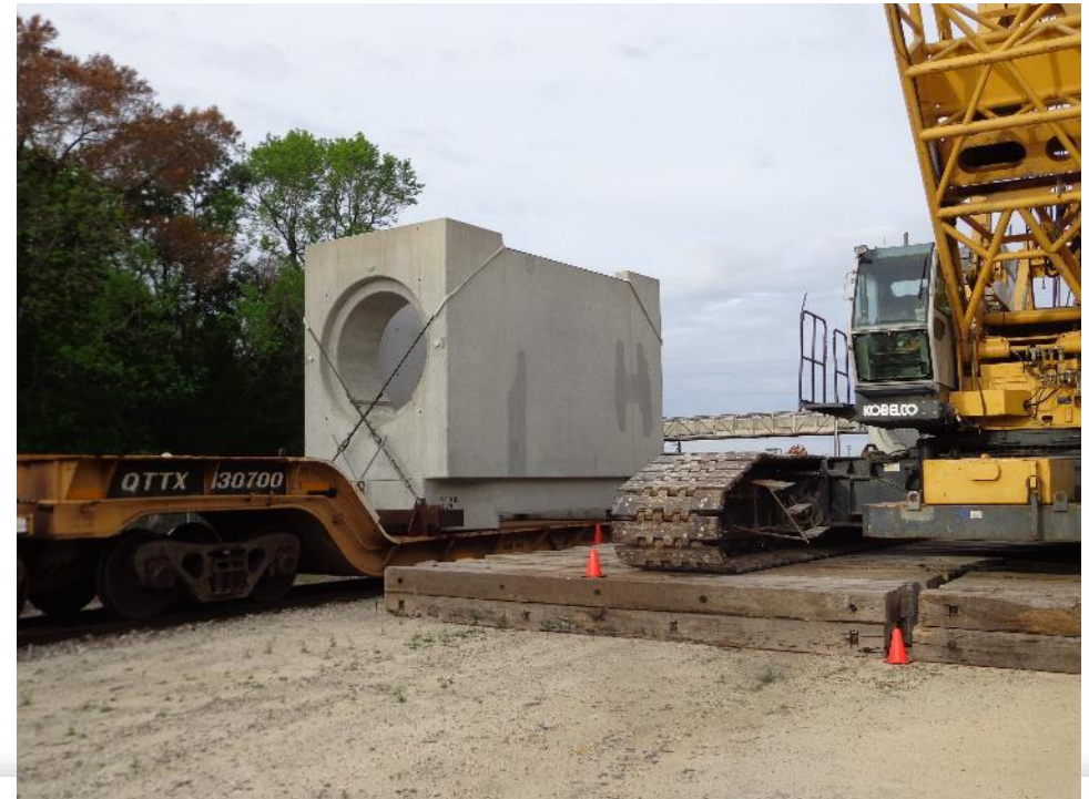
Horizontal Storage module Staged for Unloading
