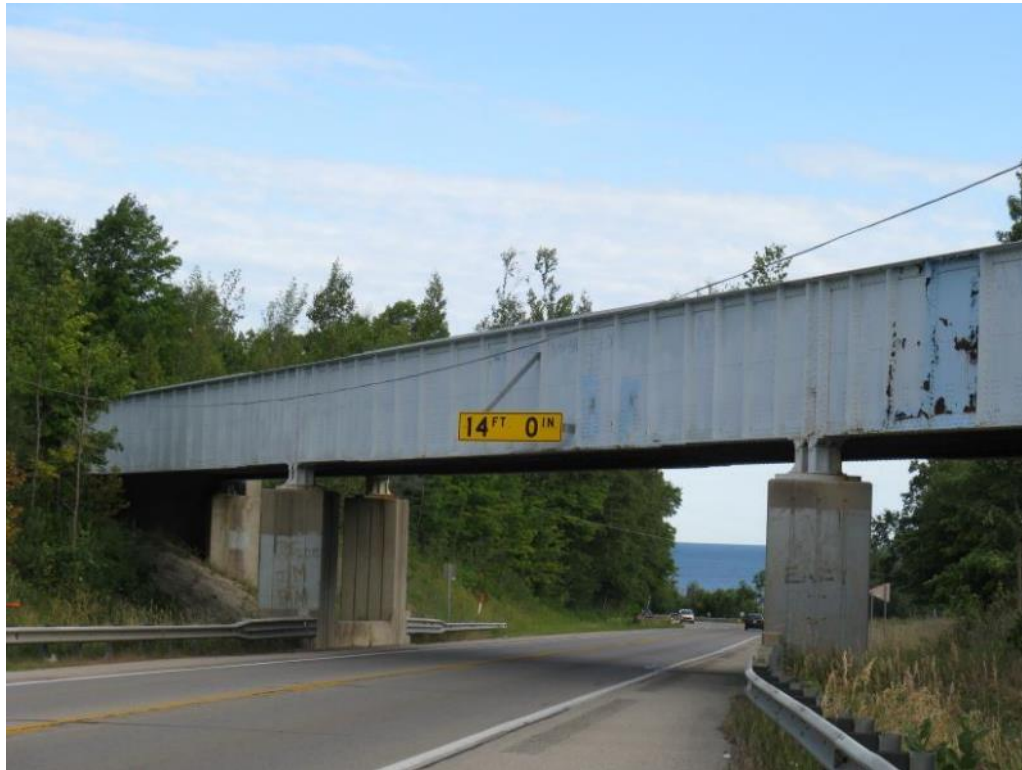
Low Overhead Bridge on U.S. 31
