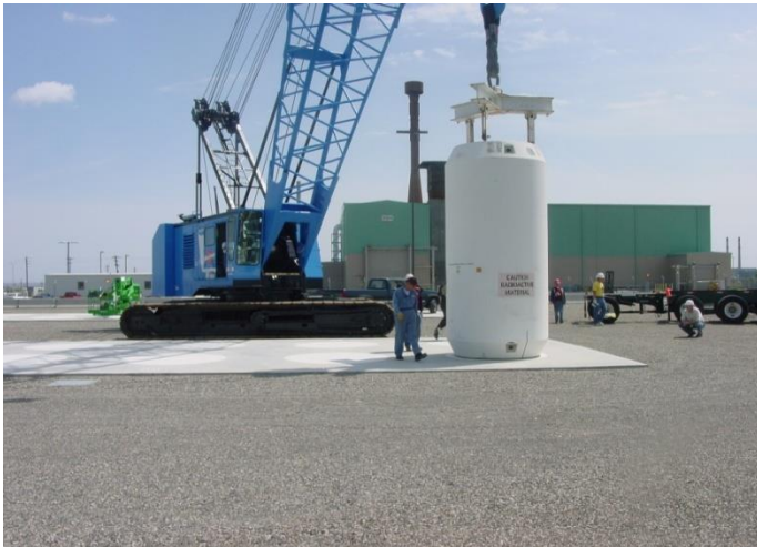
Dry Cask Storage
